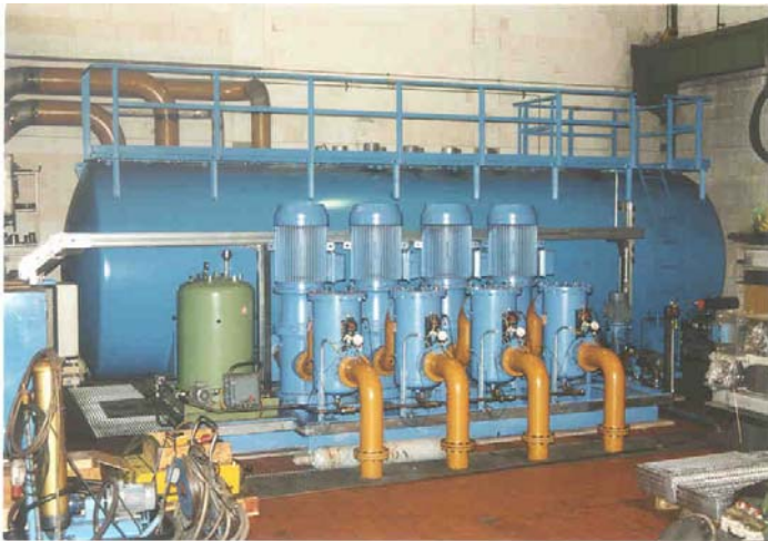
Fig. 4 New 50 m 3 tank with filling pumps and filters
