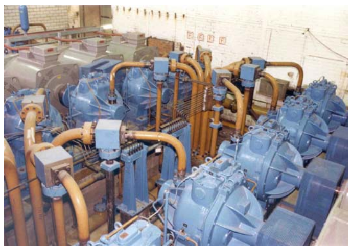
Fig. 3 Main pumps in the pump room
